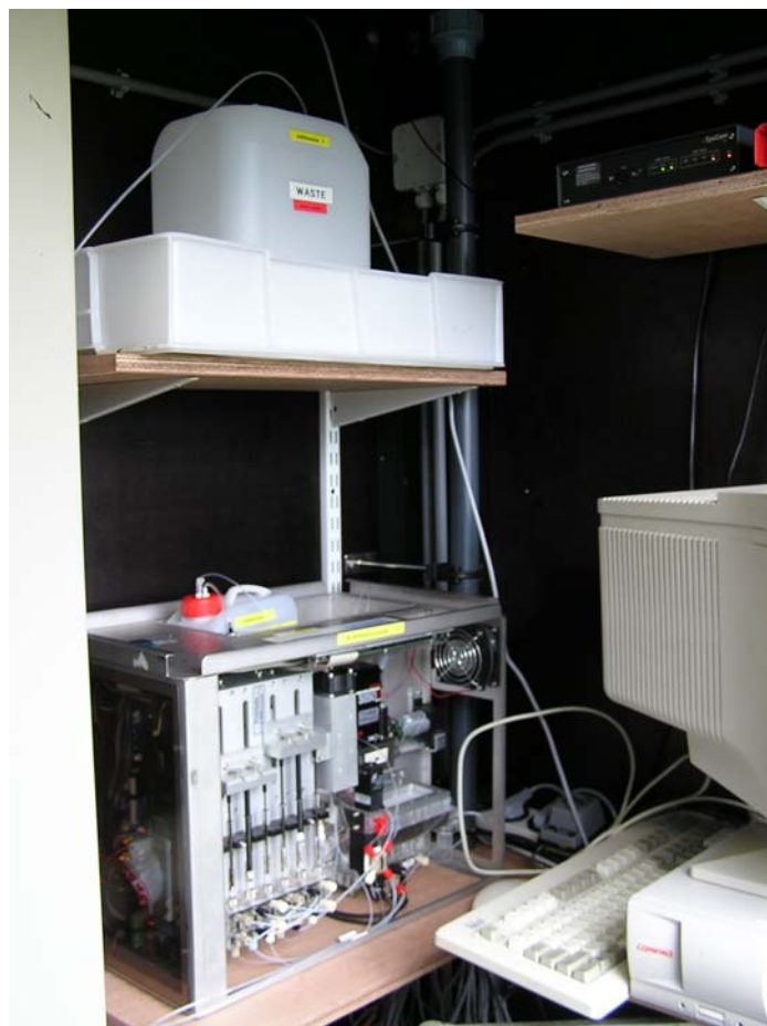
Location: Wetterskip Pumping station
